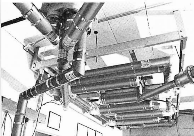
Sideband filter and notch diplexer are ceiling mounted to save space.
