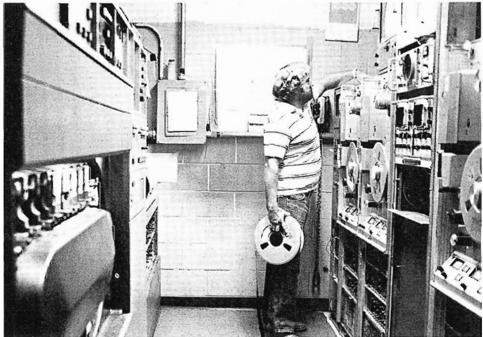
TV-4 Tape Room is compact and well-utilized.
